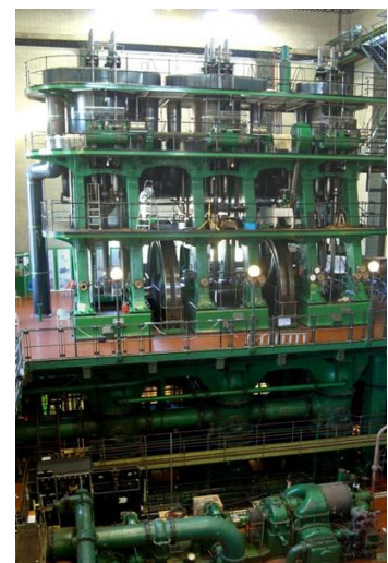
Kempton's 1000 ton triple expansion steam pumping engine
